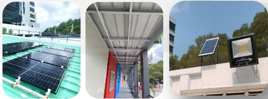
Solar panel installed at MiC office
